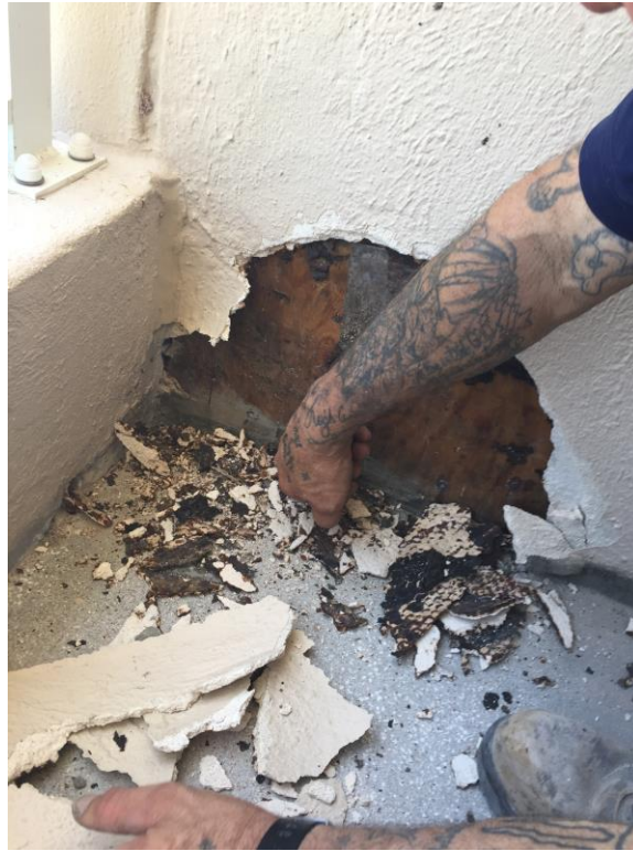
Picture 5: Unit 709 with corroded lath in stucco
